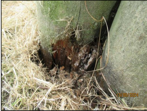
(Rotten post on net climber)
