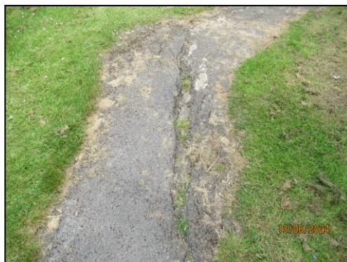
(Poor condition path)
