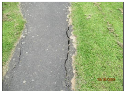
(Poor condition path)
