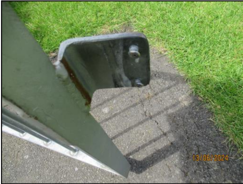
(Missing buffer at gate to play area)
