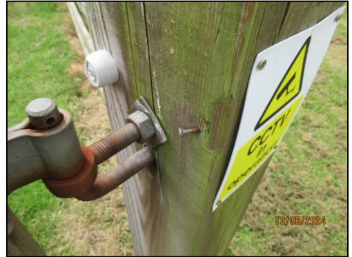
(Missing gate stop at gate to play area)
