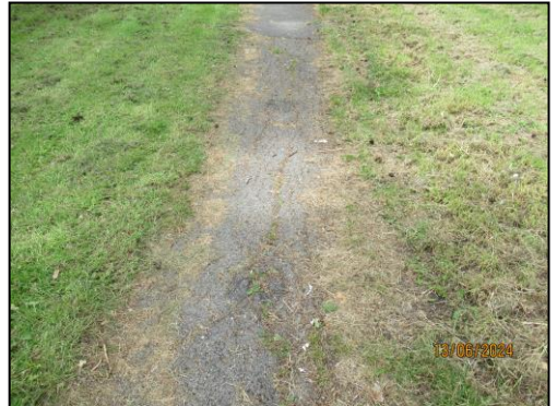
(Poor condition path)
