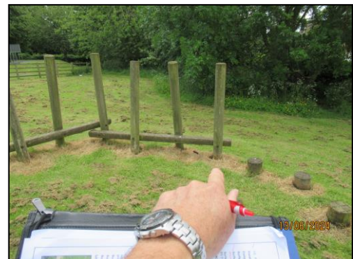
(Rotten post on weave beam)
