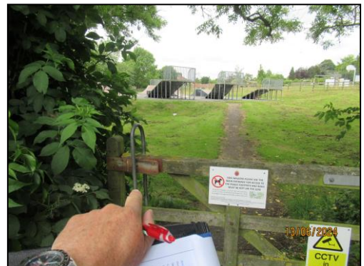
(Location of loose bracket at gate to skate park)
