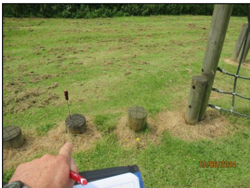
(Rotten step post)
