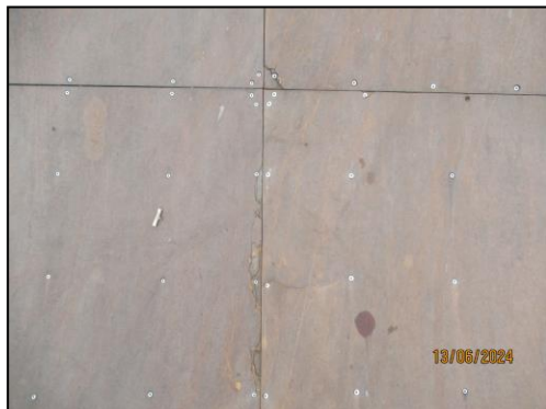
(Slight damage to liner on half pipe combi unit)
