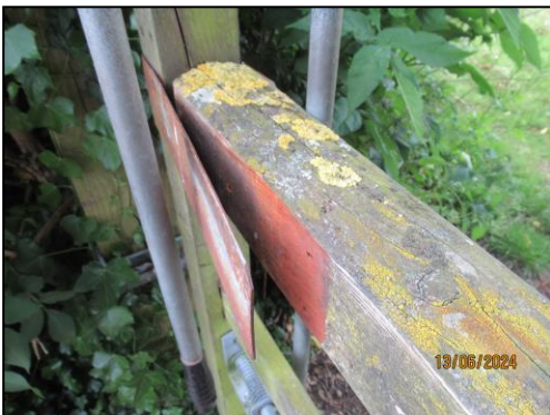
(Loose bracket at gate to skate park)
