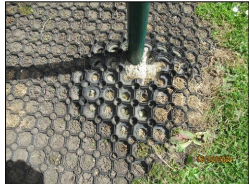
(Exposed foundations at sliding pole)
