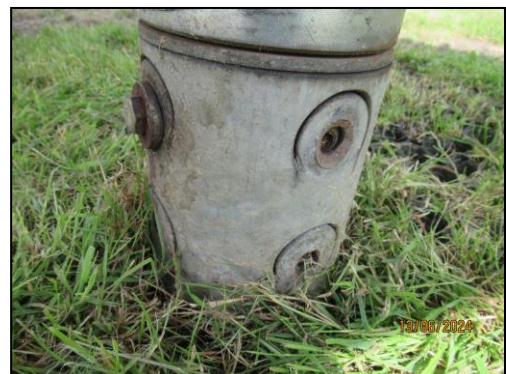
(Broken studs at ground fixing)
