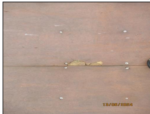
(Damaged liner on half pipe combi unit)
