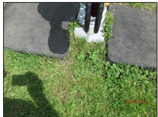
(Potential trip hazards at edges of tiles)
