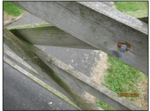
(Missing nut on bolt at gate to skate park)
